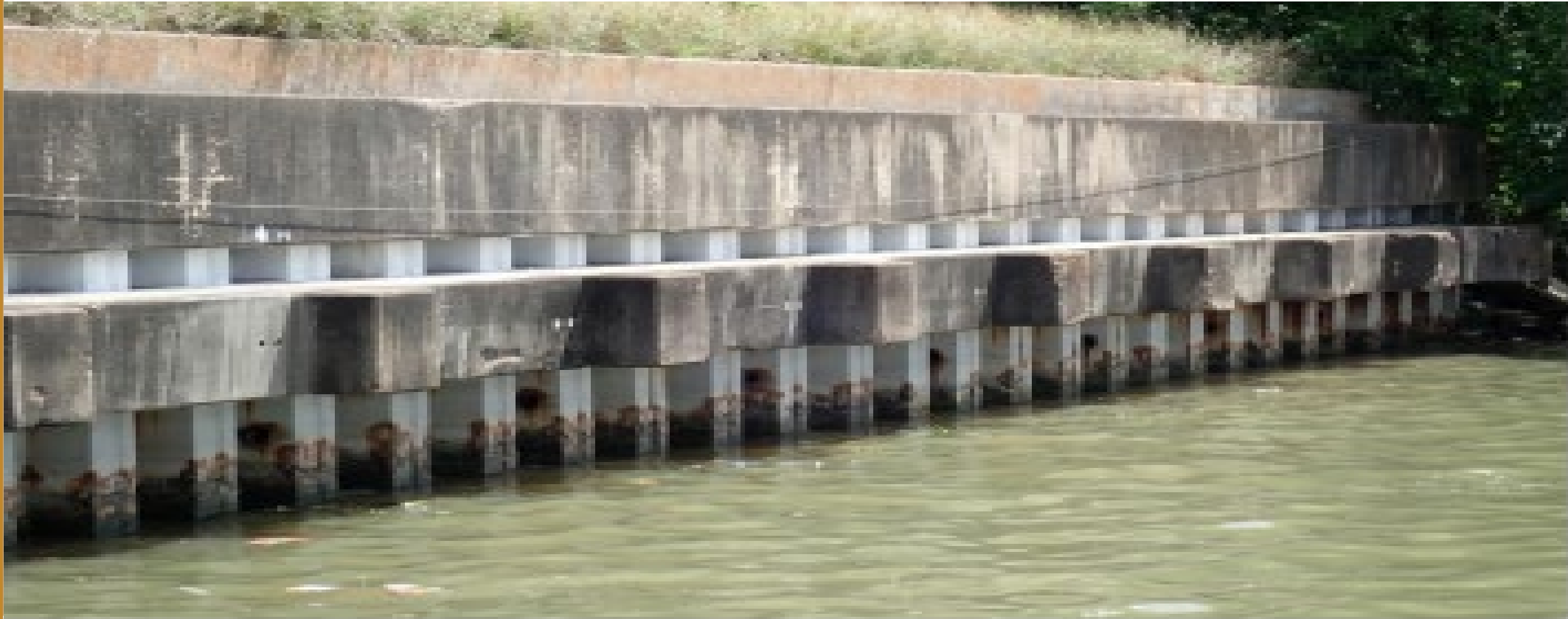
Inspection of corrosion protection systems and the condition of the assets being protected in accordance with the FICAP Corrosion program manual
